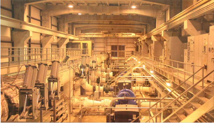
Before: High Pressure Sodium Lighting at A.B. Jewell
