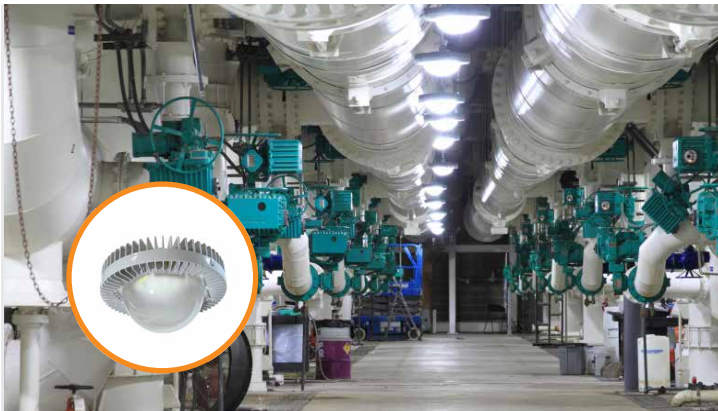
Dialight DuroSite® LED Low Bay Fixtures provide unparalleled illumination at A.B. Jewell Water Treatment Plant
